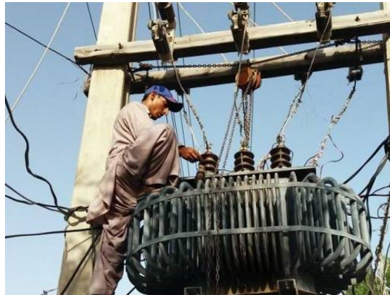
Figure1. Repair of electric transmission lines without safety measures
